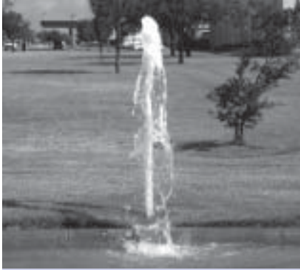
Check your system to ensure that each sprinkler head is working.
