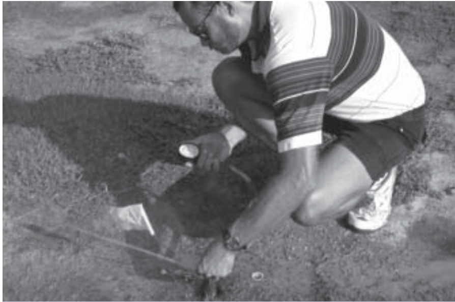
Check water pressure at each sprinkler and record pressure problems.
